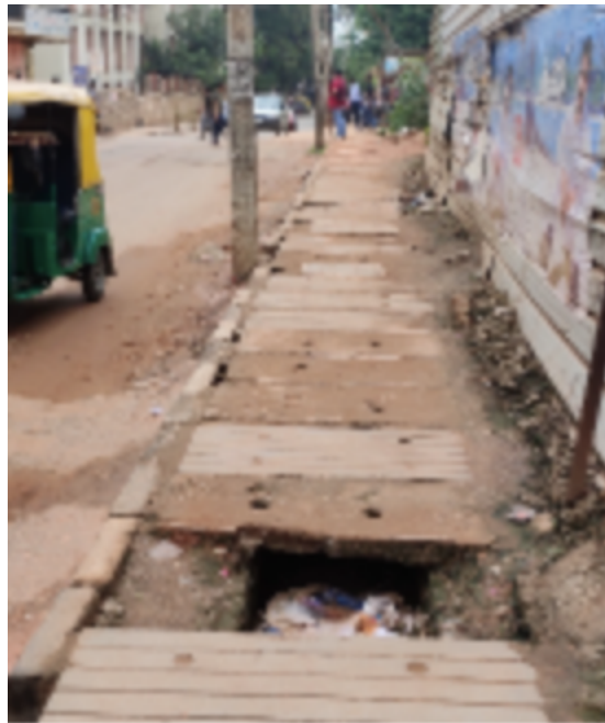
2.0: Footpaths condition is good except minor obstructions, cracked or missing panel, minor overhead hazards, one to two detours.
